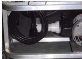
Cooling System Power Cord
